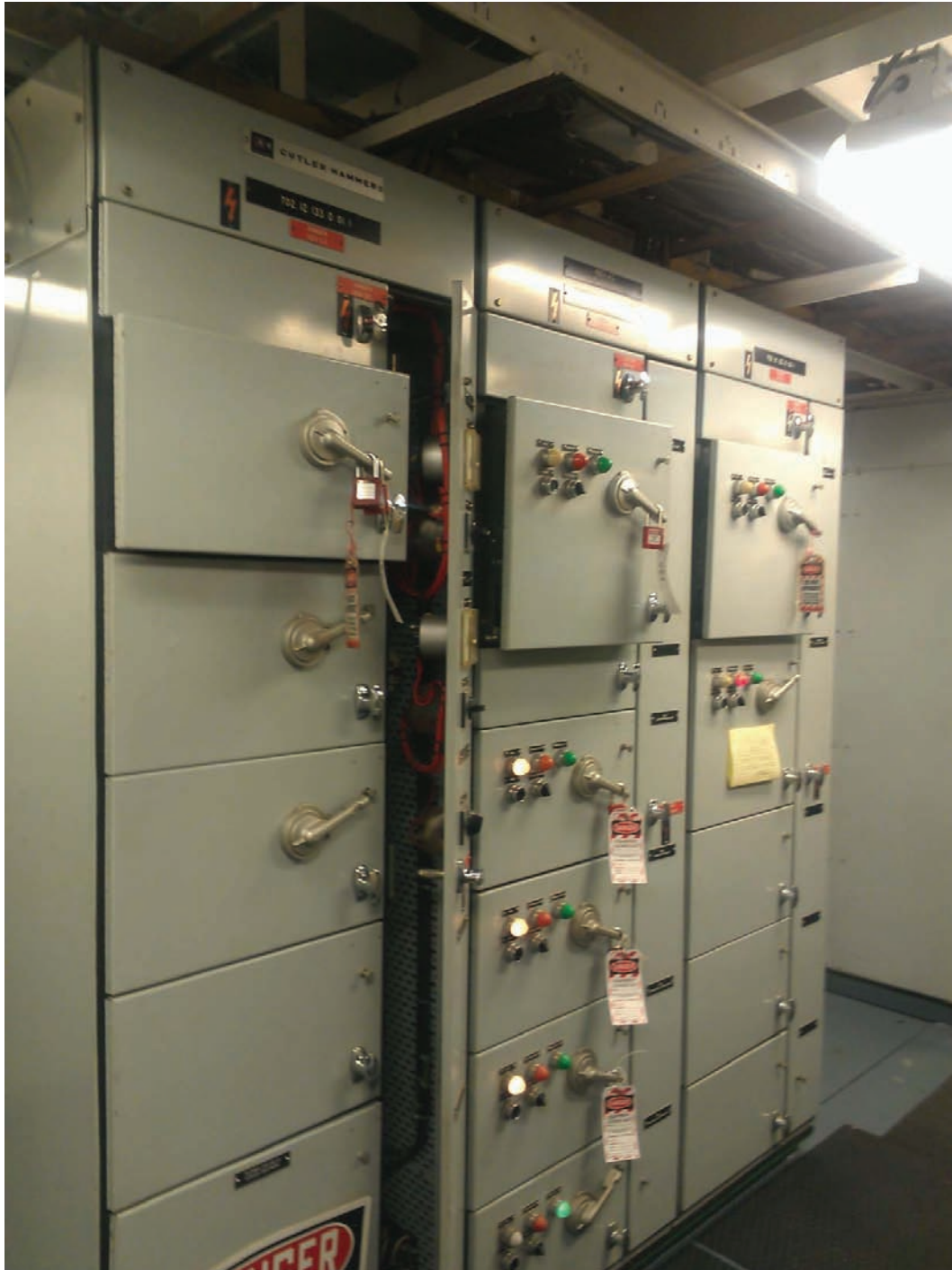
Photograph 3: 480V Motor Control Center
