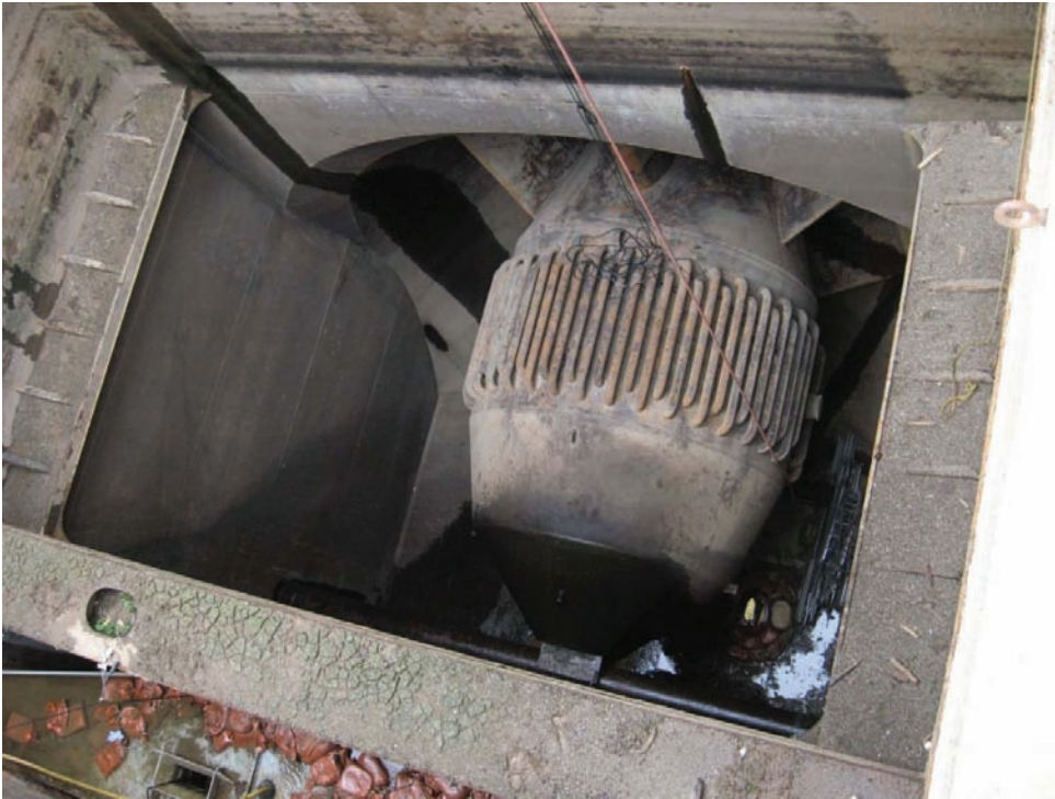
Photograph 4: Generator Cooling System Piping
