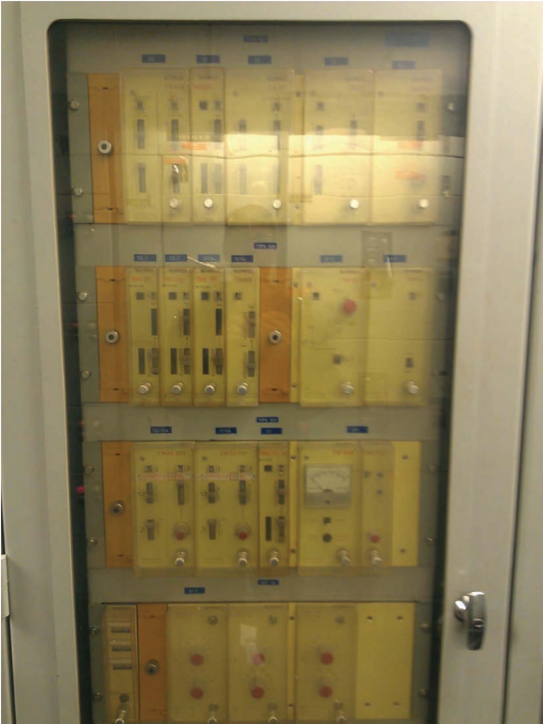
Photograph 2: Turbine Governor Panel
