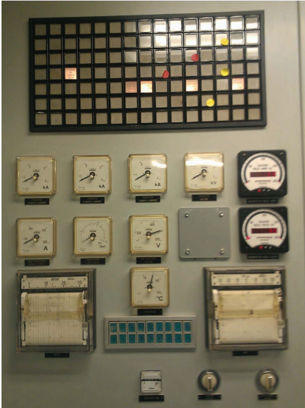
Photograph 1: Control Room Panel
